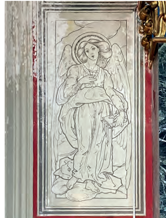
Damage from water ingress to original Art Nouveau sgraffito decoration.
