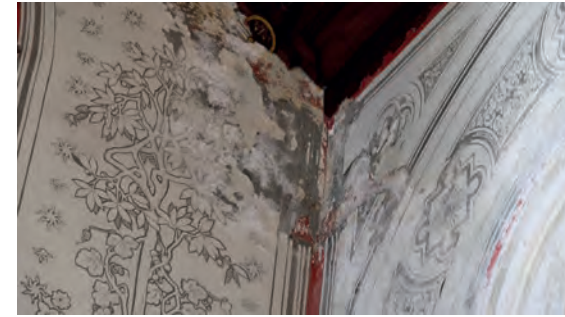
Water damaged sgraffito , Church of the Ascension.
